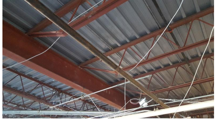
Figure 6: Heavier black piping which must be installed overhead.
