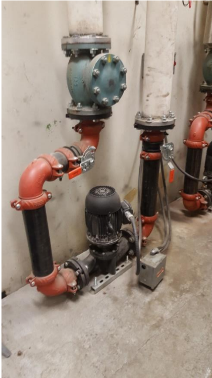
Figure 5: Valves and fittings installed.
